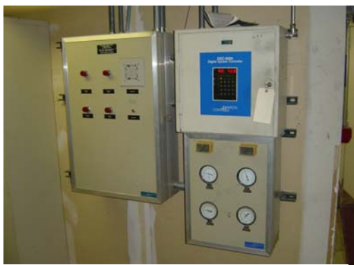
A newer DDC control panel adjacent to original pneumatic control panels
