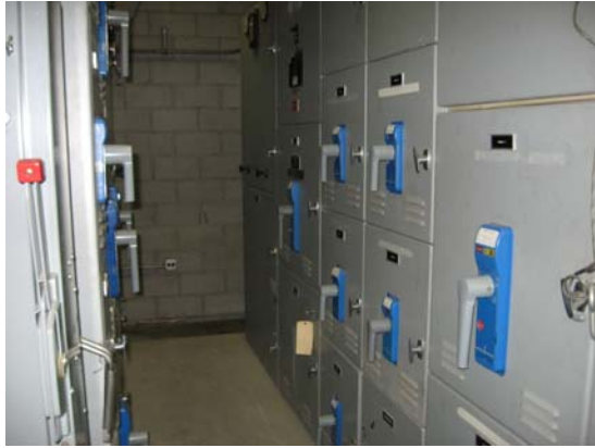
Main Building Switchgear Lineup
