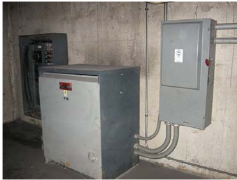
Obsolete Mechanical Room Equipment
