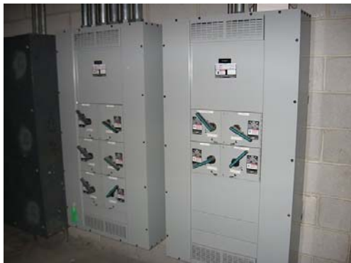
Newer Electrical Distributed Equipment
