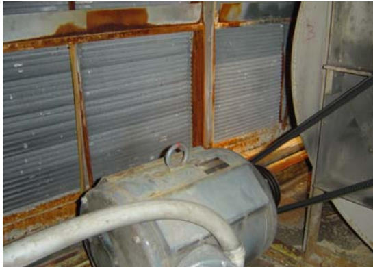
Significant corrosion and deterioration in air handling unit fan section
