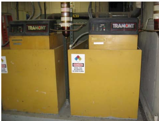
Existing Generator Day Tanks
