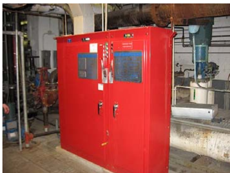
Main Fire Pump Controller
