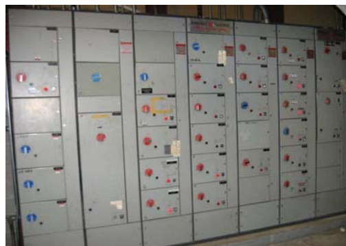
Obsolete Motor Control Center
