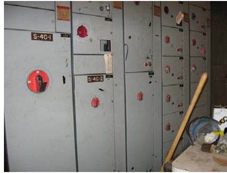
Obsolete Motor Control Center
