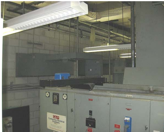
Switchgear Breaker Winch Assembly
