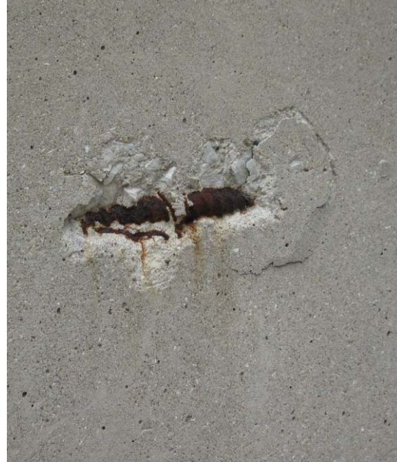
TT Photo #4: Exposed rebar due to concrete spalling
