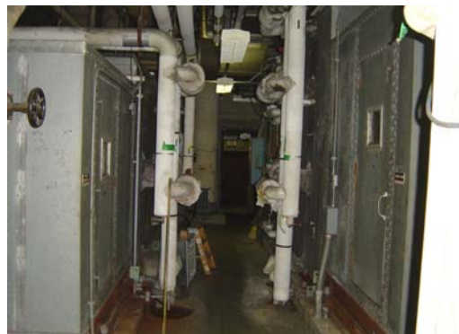
Maintenance Area is extremely limited in many areas of existing Prentice
