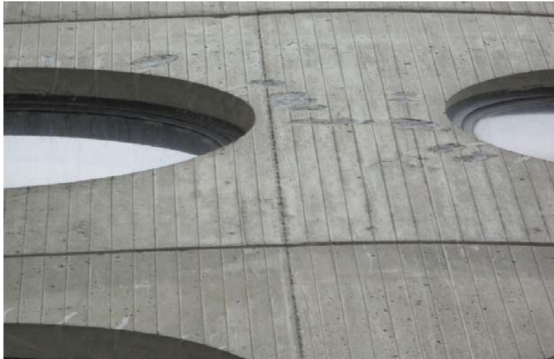
TT Photo #1: Concrete spalling at exterior wall
