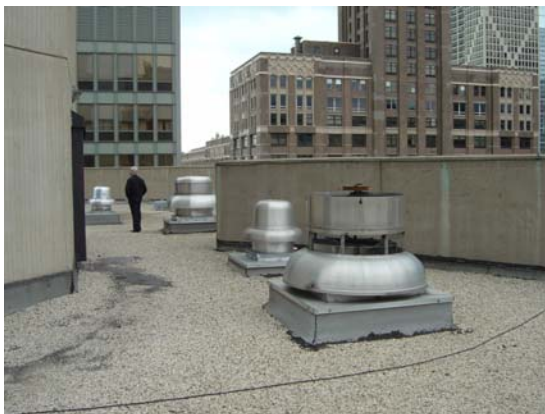
Roof Fans on Existing 5 th Floor – Exhaust Air is required to be Re-Directed to the Roof
