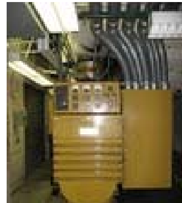
Existing Emergency Generators
