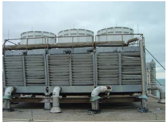
900 ton Cooling Tower located on the Prentice Roof
