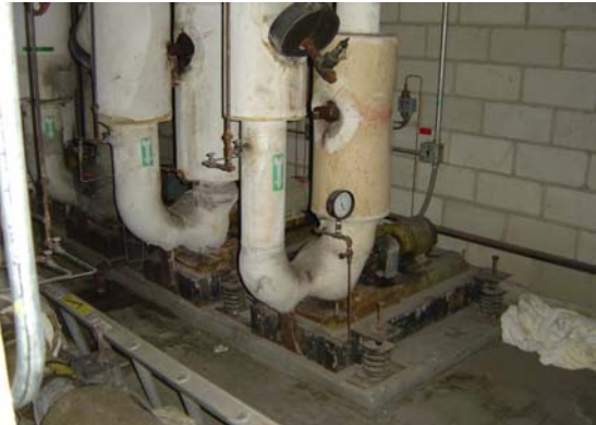
Worn and Corroded Pumps
