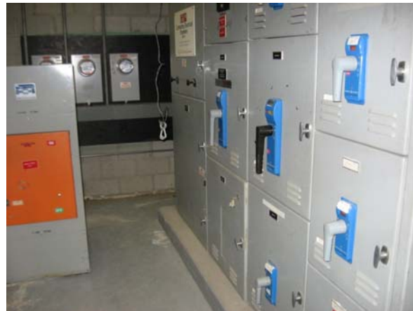
Main Building Switchgear Lineup
