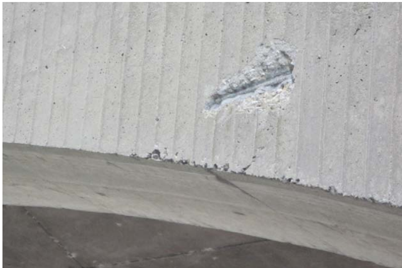
TT Photo #2: Exposed rebar due to concrete spalling
