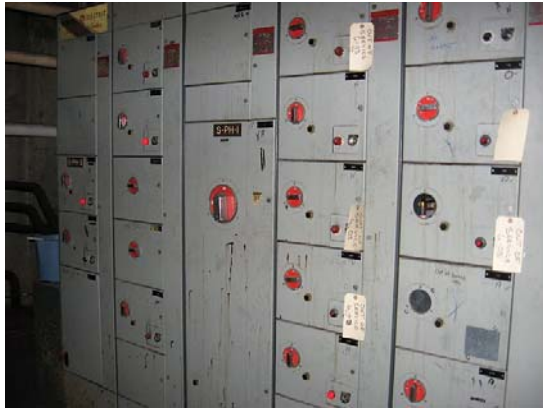
Deteriorated Motor Control Center
