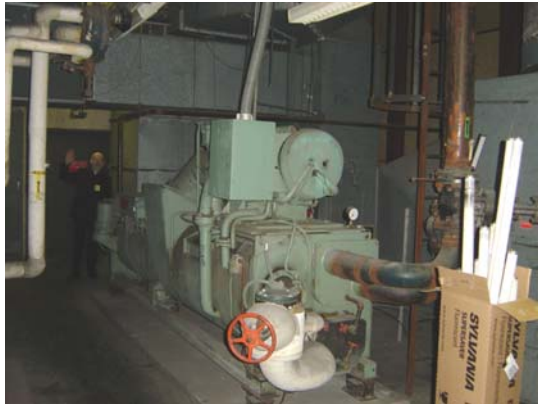
One of two 900 ton chillers located in the Basement Equipment Room
